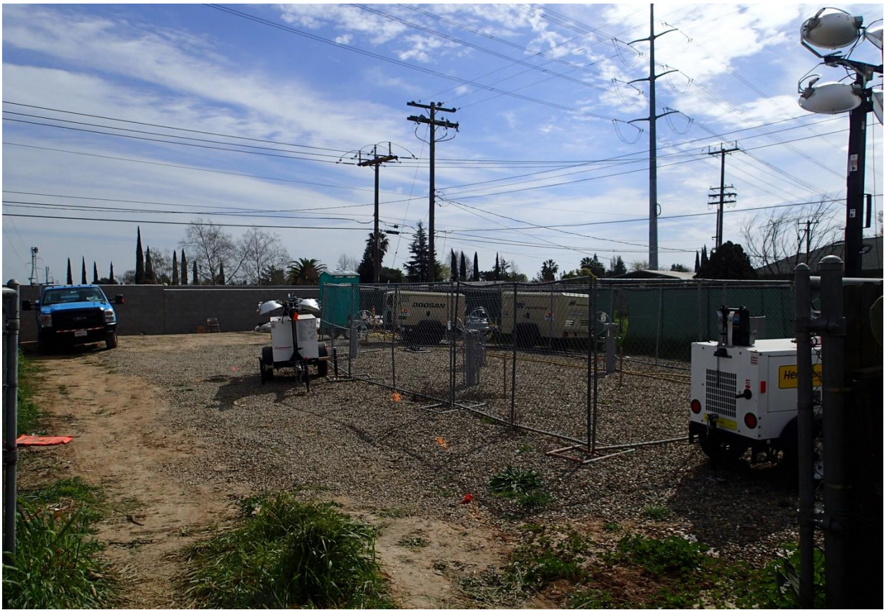
Photo 3: View of the PG&E valve lot facing east. The Blue Line LRT tracks lie immediately beyond the soundwall in the background, and the backyard of the Meza property lies to the right behind the fence shown in the photo.
