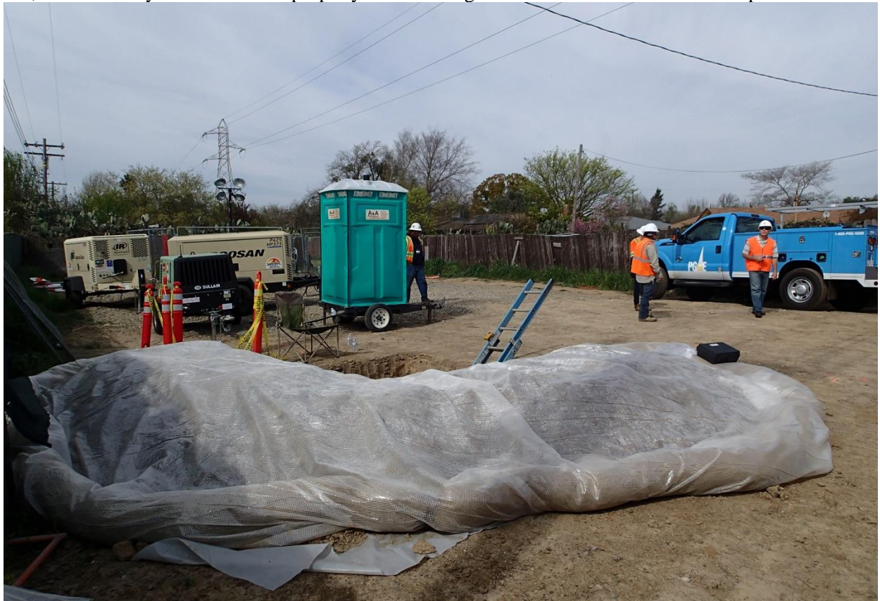
Photo 4: View of the PG&E valve lot facing northwest. The Meza property lies to the immediate left of the photo.
